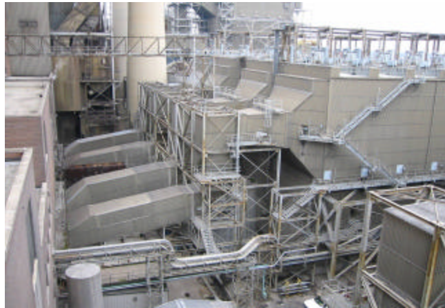
Figure 11. Ductwork leading to the St. Clair ESPs.
